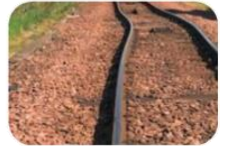
Heatwaves can cause track to buckle
