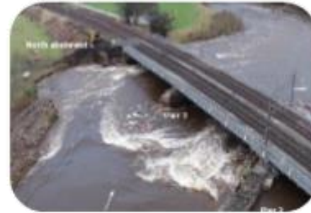
Flooding can cause erosion, destabilising bridges
